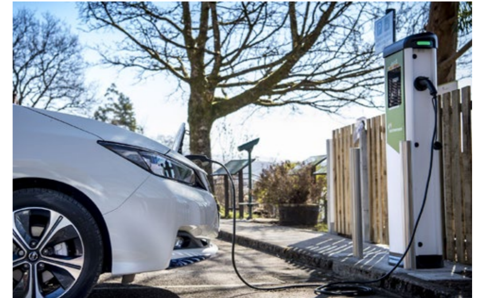
Fig. 22 - Electric vehicle charging point.
