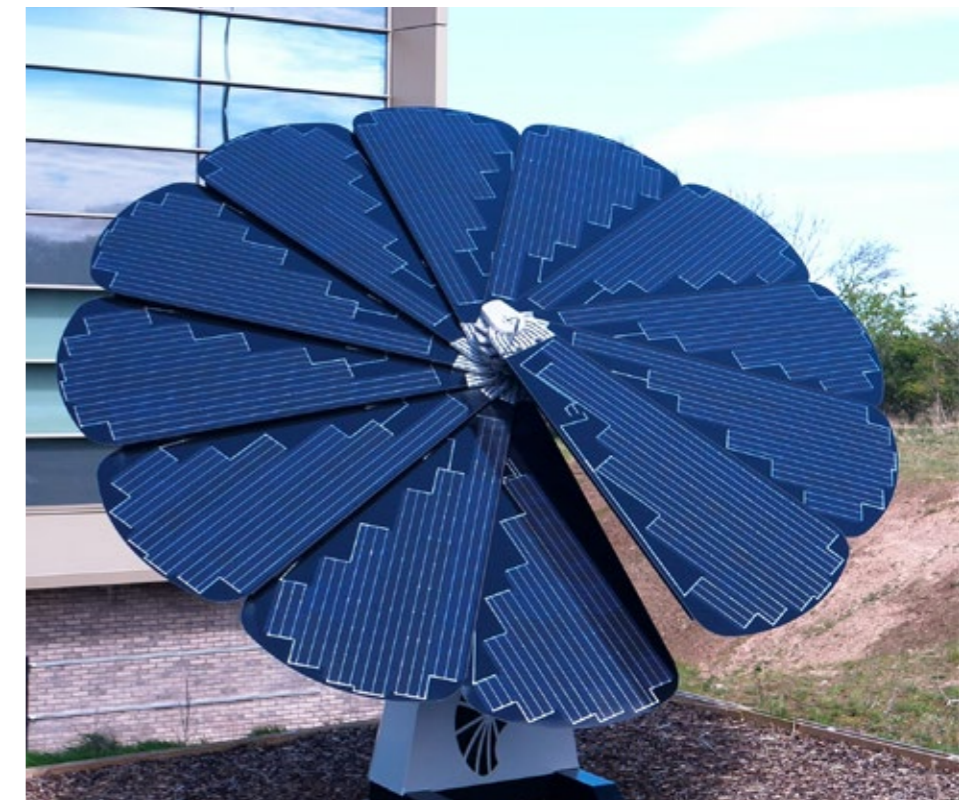
Fig. 24 - Existing solar panels installed on SEZ site.
